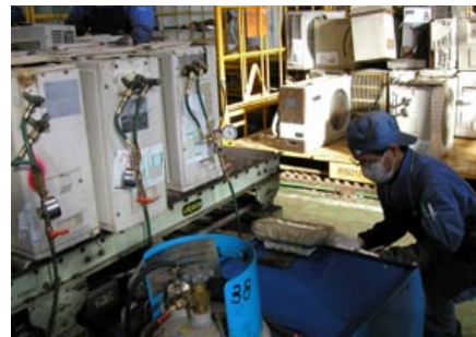
Refrigerant fluorocarbons are recovered by dedicated equipment. Recovered fluorocarbons will be destroyed at designated treatment facilities.
